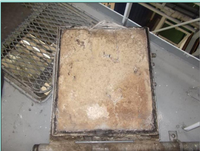
Doors found in very poor conditon
