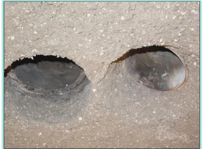
Guide tubes for burners in roof.
