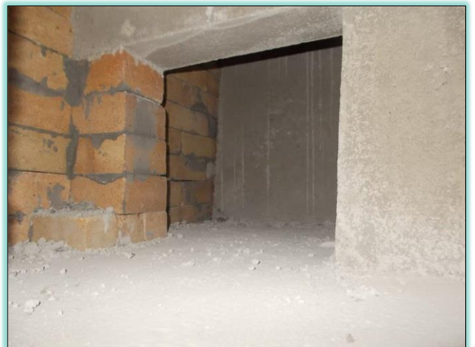
View into second chamber through third chamber. Note the heavy beam casted in place
