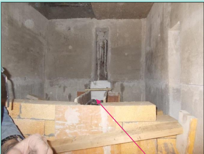
Dividing wall in first chamber. Note the heavy support beam being casted
