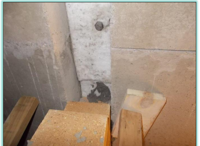
Wall securely anchored inside wall. Note the ceramic fiber insulation to casing
