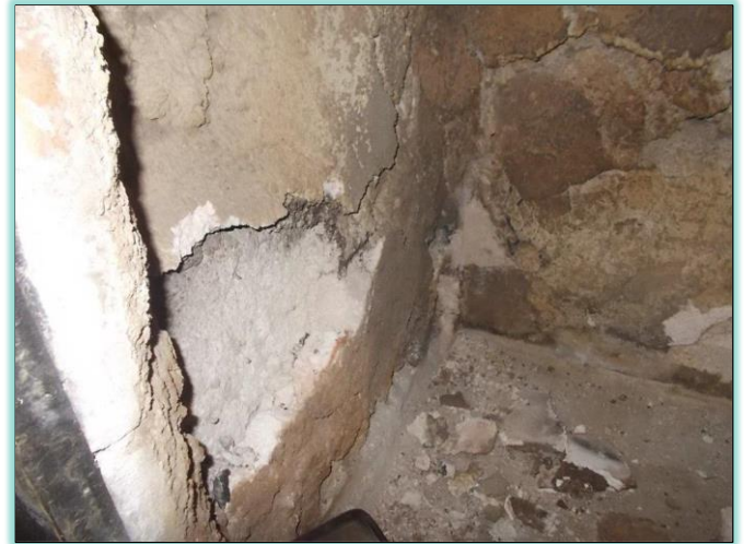
Internal condition found quite miserable
