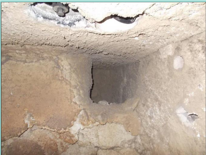
Dividing wall to second chamber found close to collapsing (note burners in roof)
