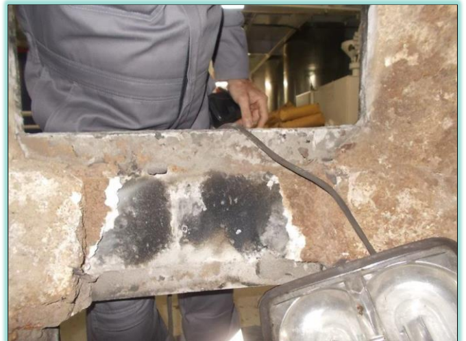
Front wall casing disposed to the heat with risk of damage
