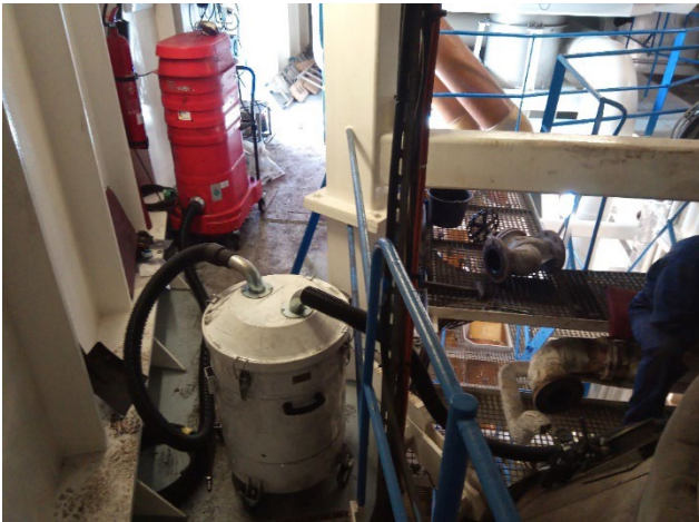
Figure 8 Vacuum cleaner with cyclone separator to minimize downtime while cleaning
