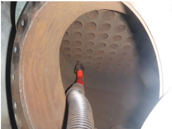
Figure 4 Cleaning of vertical fire tubes from the bottom part of the boiler
