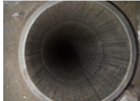
Figure 9 Tube condition after cleaning
